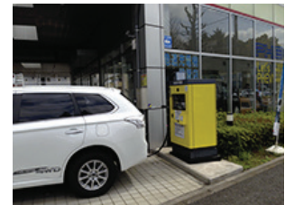
Quick charger installed in a dealer
