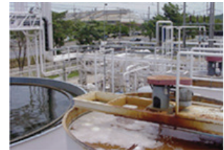
General effluent treatment facilities
